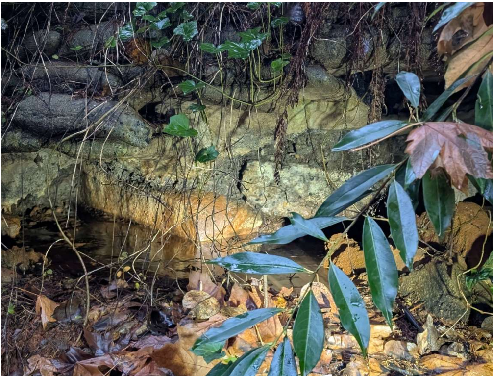
Photograph 2 – Undermined Fill Bags (Looking northeast).
