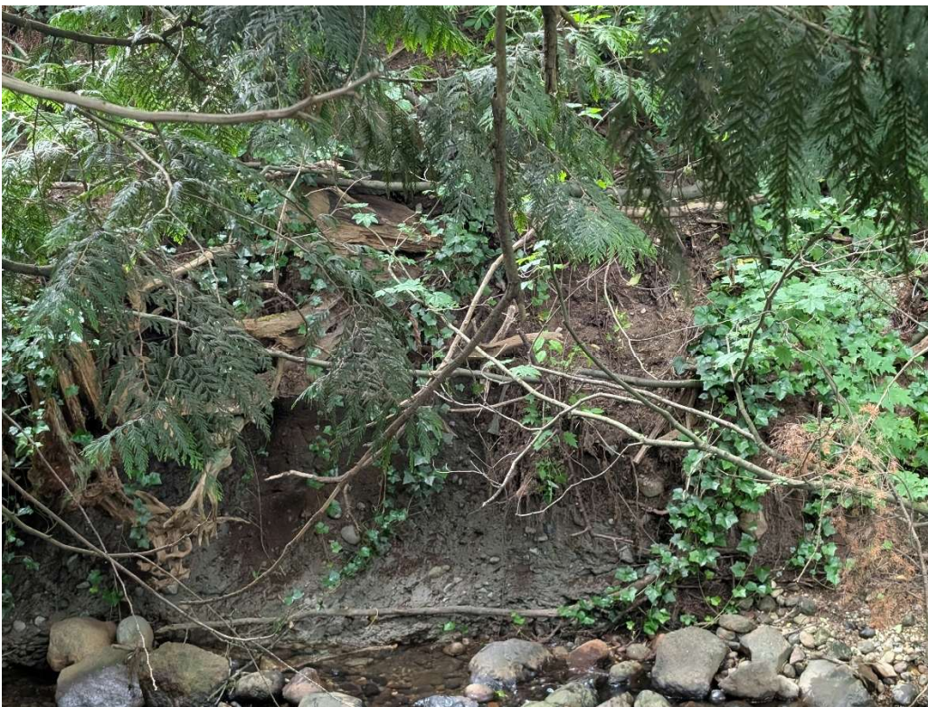
Photograph 2 – The eroded toe of the ravine slope (Looking west).
