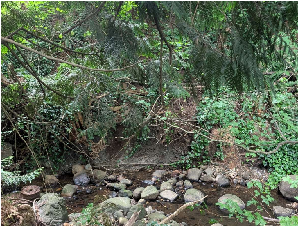
Photograph 1 – Overview of the west ravine slope and the eroded toe (Looking west).
